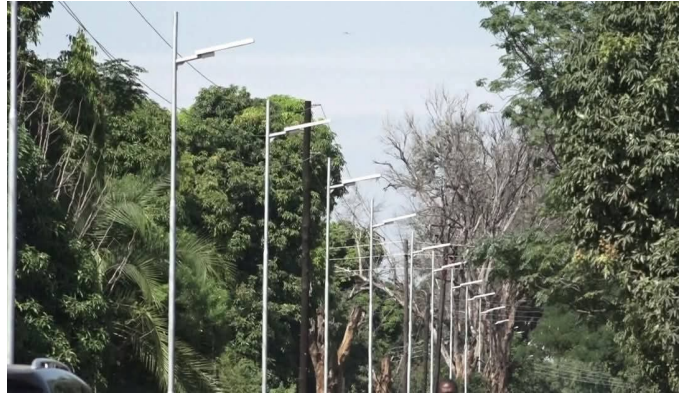
Newly installed street lights
