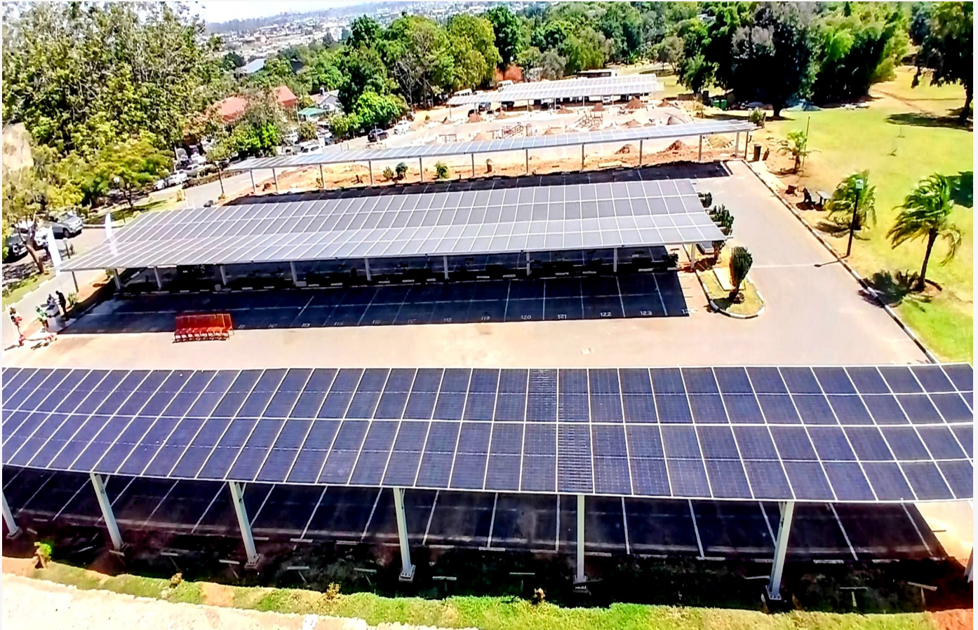
The commissioned 750-kilowatt Solar photovoltaic (PV) Plant at Parliament Buildings.
