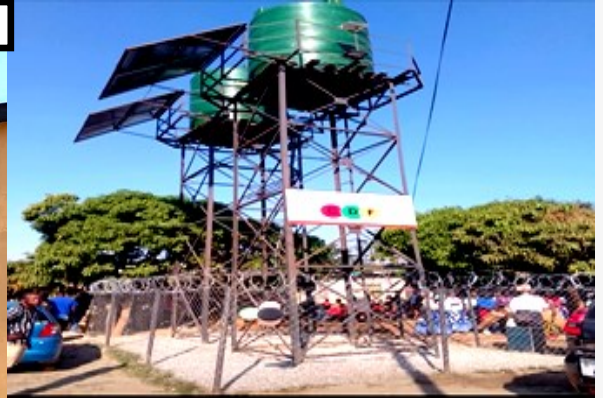
The Chunga Water Reticulation System in Chunga Ward.
