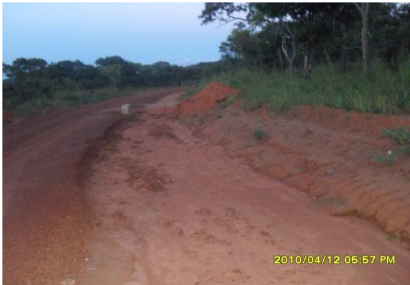
Parts of the Kasama-Safwa-Chinsali Road washed away by heavy rains
