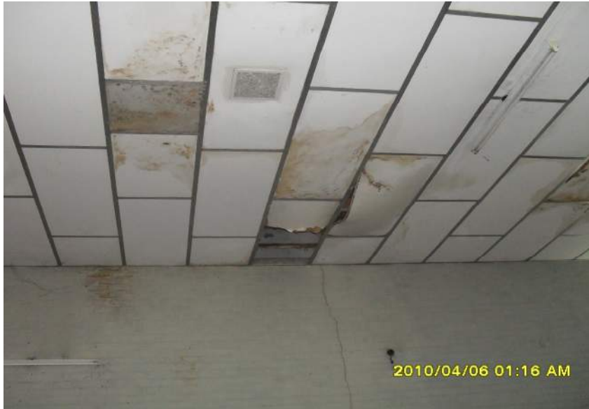
Dilapidated Ceiling Board at NCH Lecture Theatre
