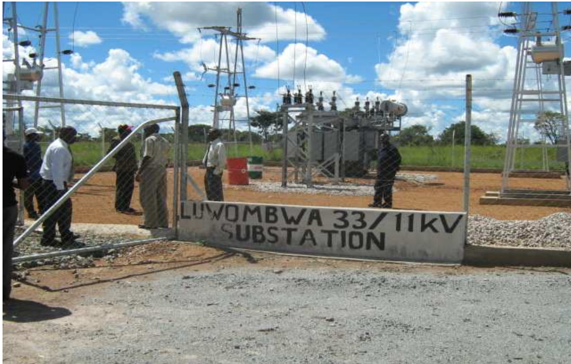
Luwombwa substation to supply electricity to Nansanga farm block
