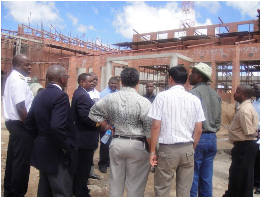
Part of the One Stop Border Post building under construction in Nakonde
