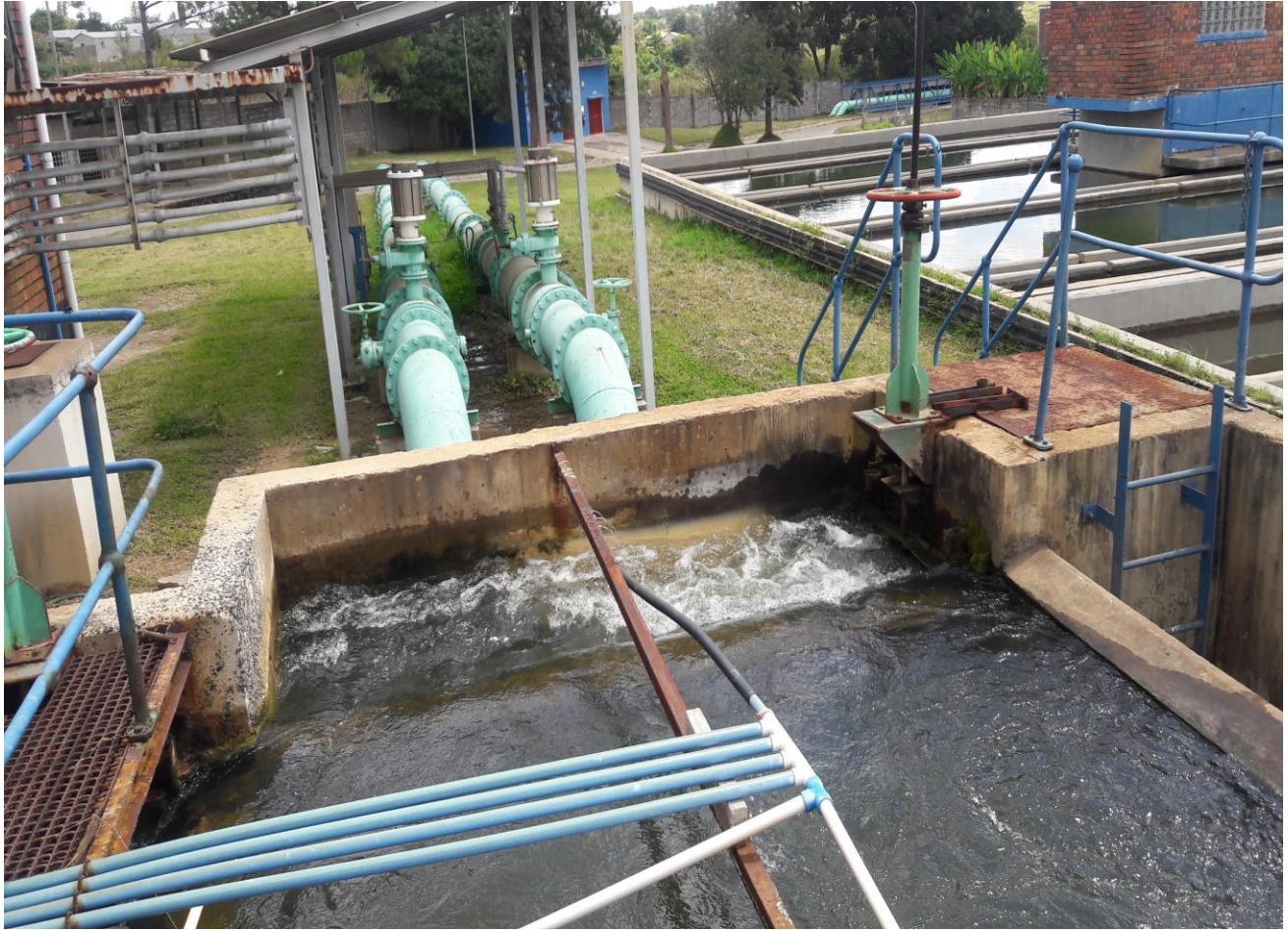
Bulangililo Water Treatment Plant – Nkana Water and Sewerage Company
