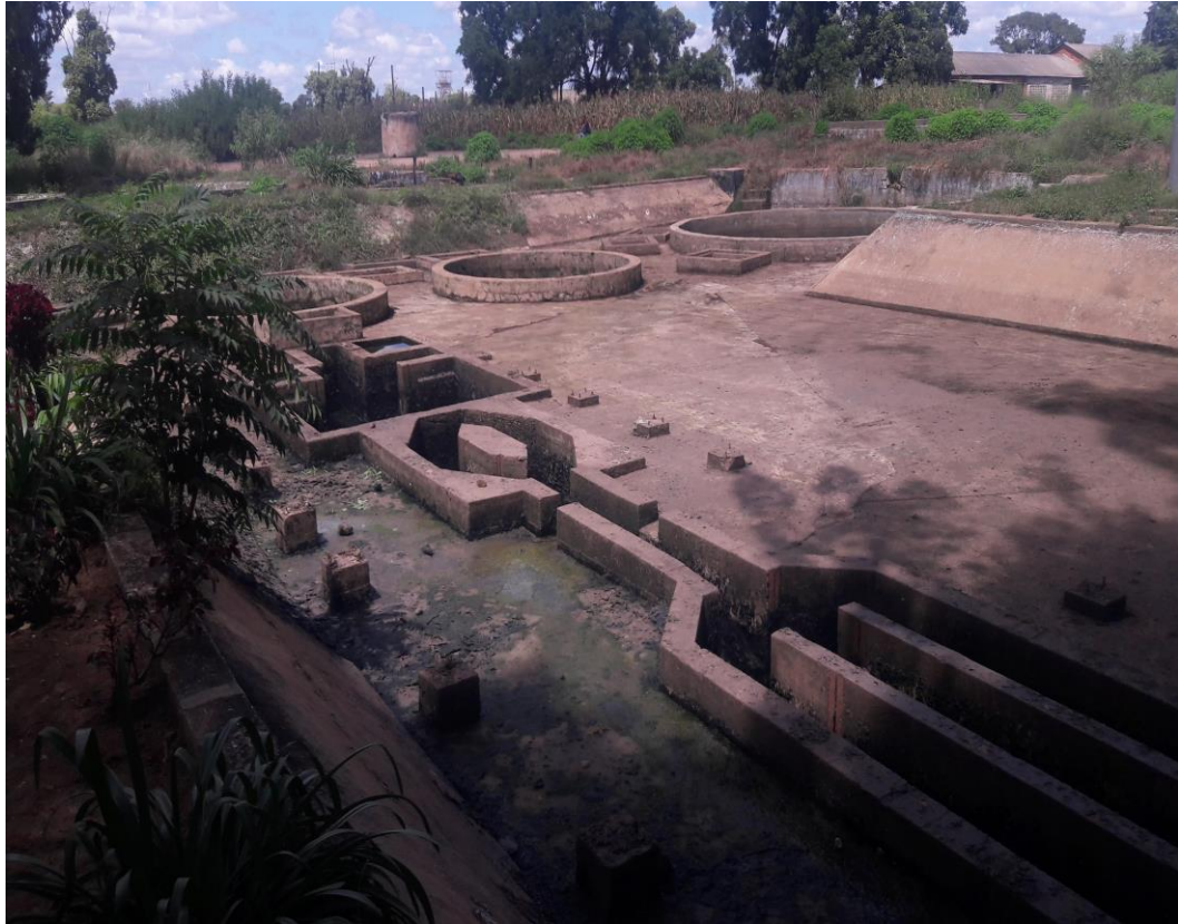
Kasanda Sewerage Treatment Plant – Lukanga Water and Sewerage Company
