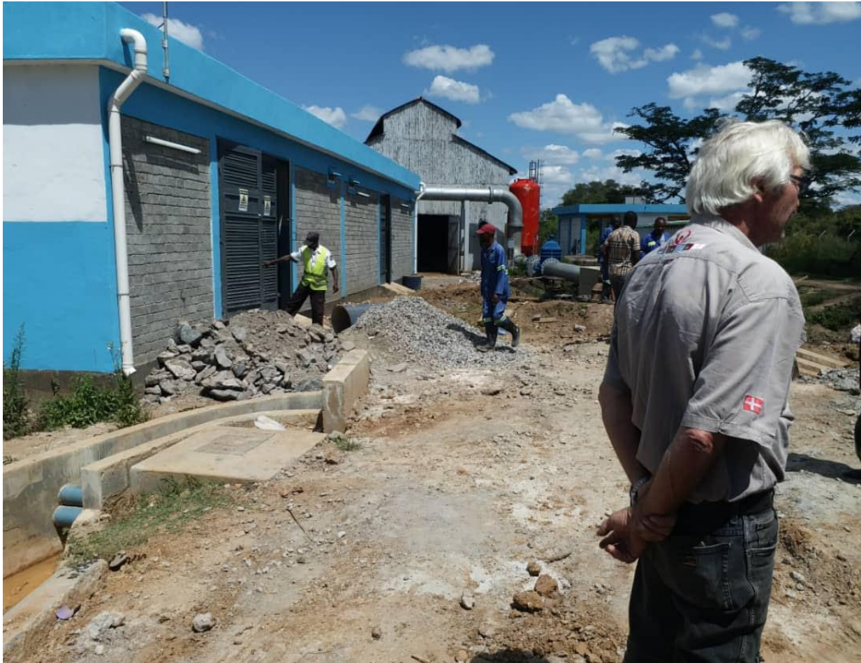
Kafubu Intake/Compact Treatment Plant – Kafubu Water and Sewerage Company
