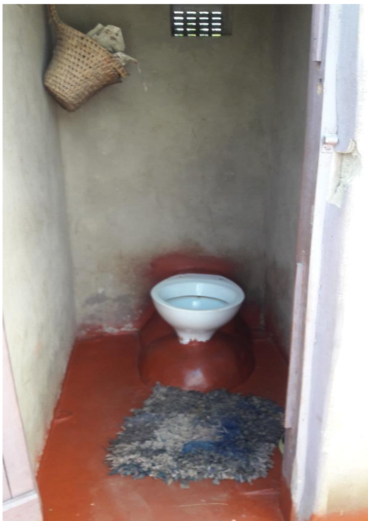
VIP Toilet, Ipusukilo - Nkana Water and Sewerage Company
