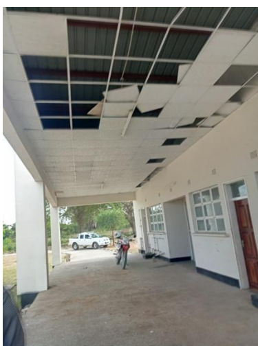
In Picture: depicting the falling ceiling at the Administration Block
