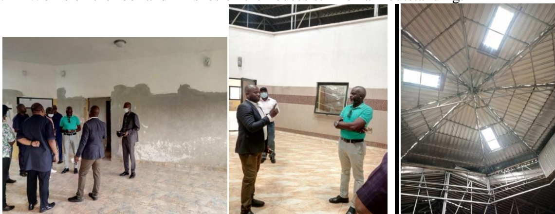
Members of PAC inspecting renovation works on the houses and the uncompleted roofing at the Mission building in Abuja, Nigeria
