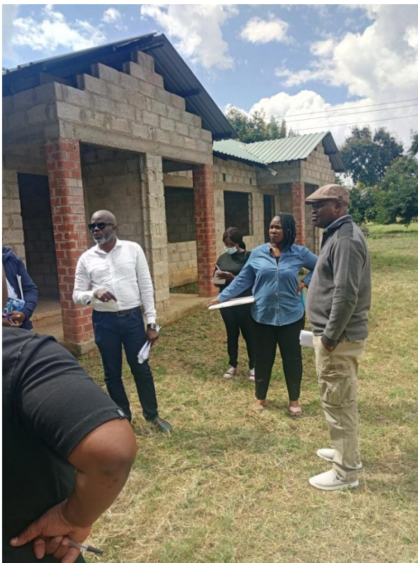
In Picture: Members of Public Accounts Committee led by Mr W C Mwambazi, MP engaging the Contractor on site
