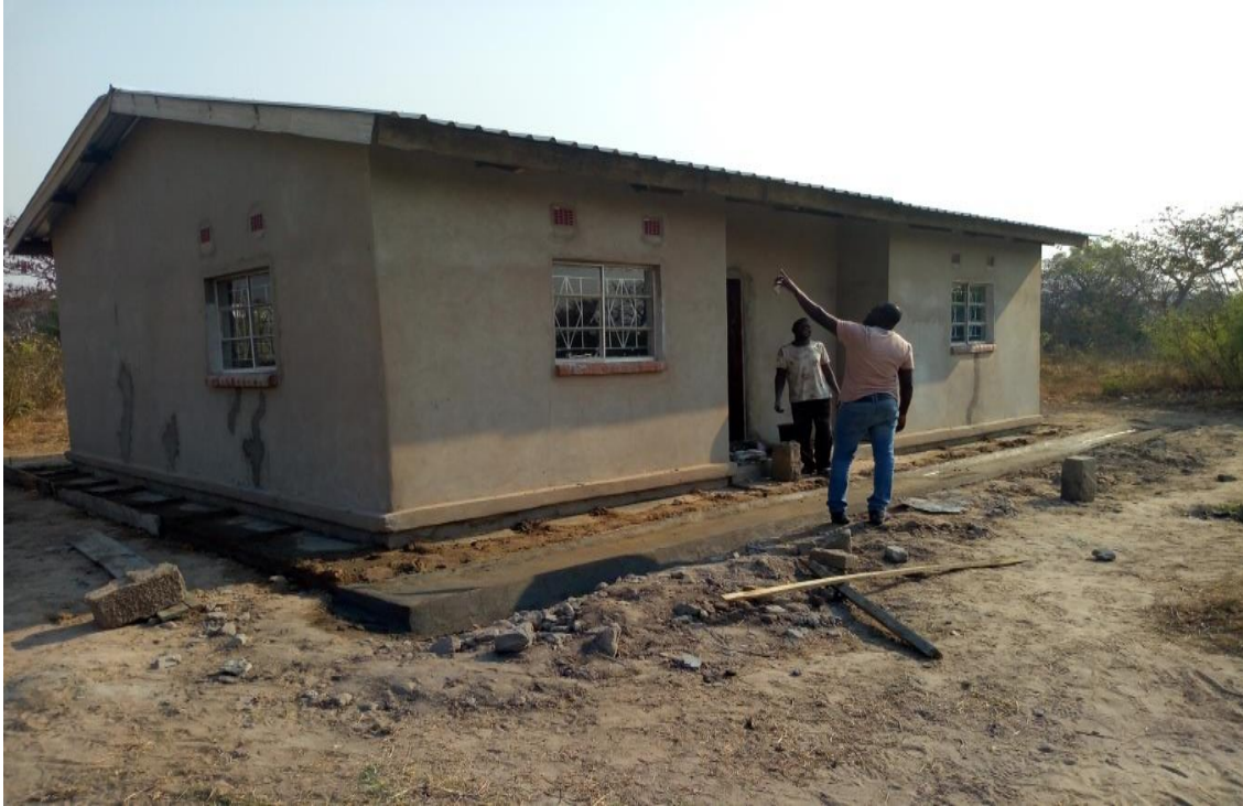
Fig: Showing Status of Staff House at Buunga Health Post in Itezhi-Tezhi District.
