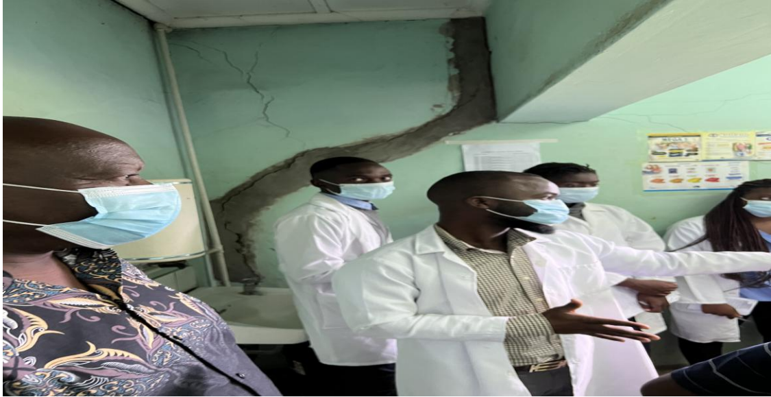
Cracking in the condemned orthopaedic workshop building at KTH
