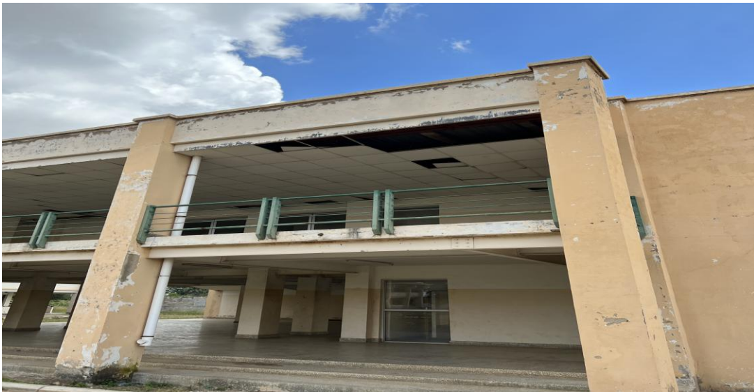
Dilapidated ceiling board at the new wing
