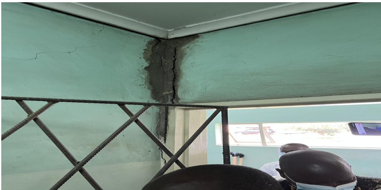
Cracks in the orthopaedic workshop/clinic
