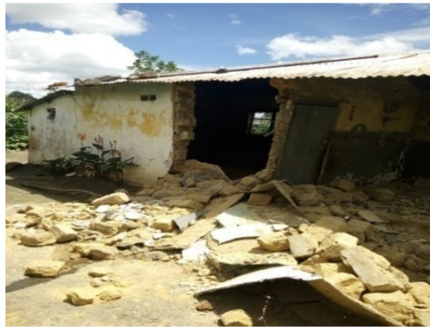
Examples of deteriorating houses in Roan Township, Luanshya, which were visited by the Committee
