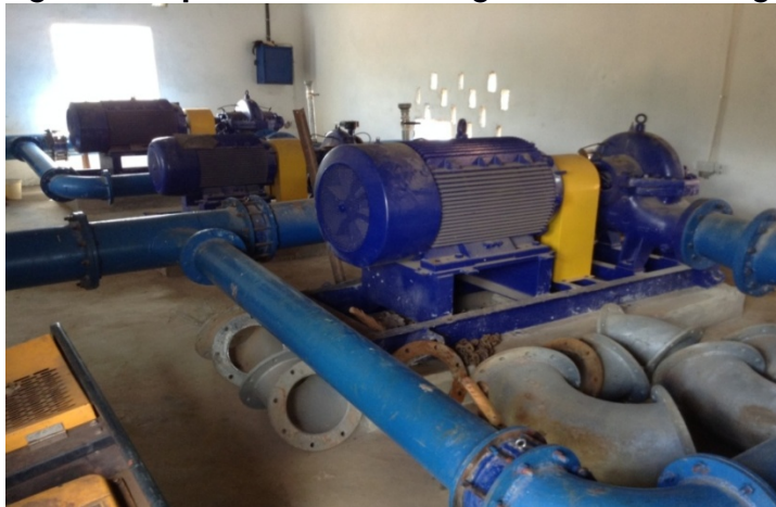
Fig.18: Pump station at Nansanga Correctional Irrigation Site
