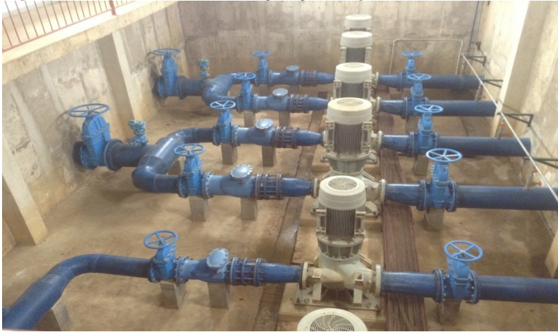
Fig. 2: Pump Station at Manyonyo Irrigation Scheme
