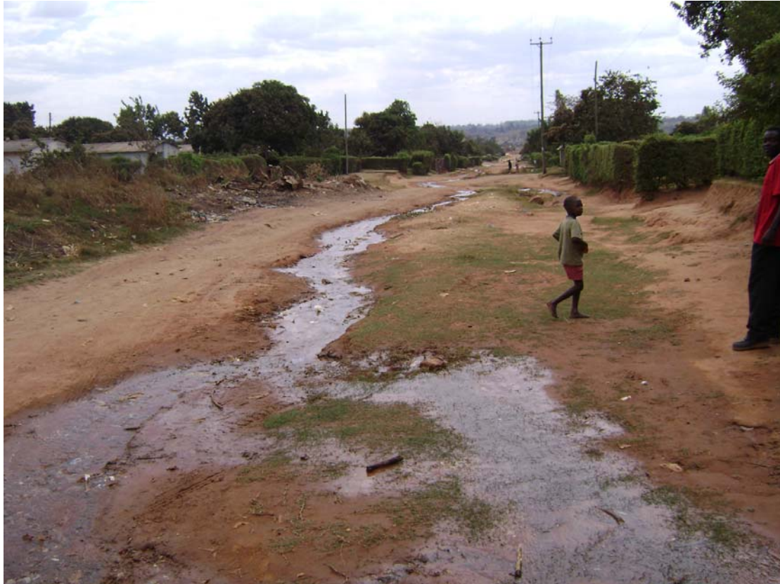
A deteriorated road in Mushili Township - Ndola
