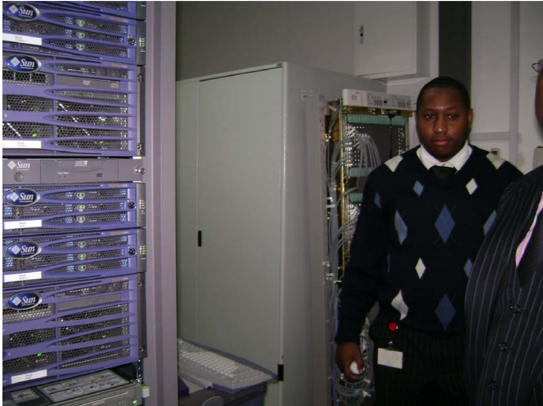
State of the Art Switch Room at Celtel Zambia
