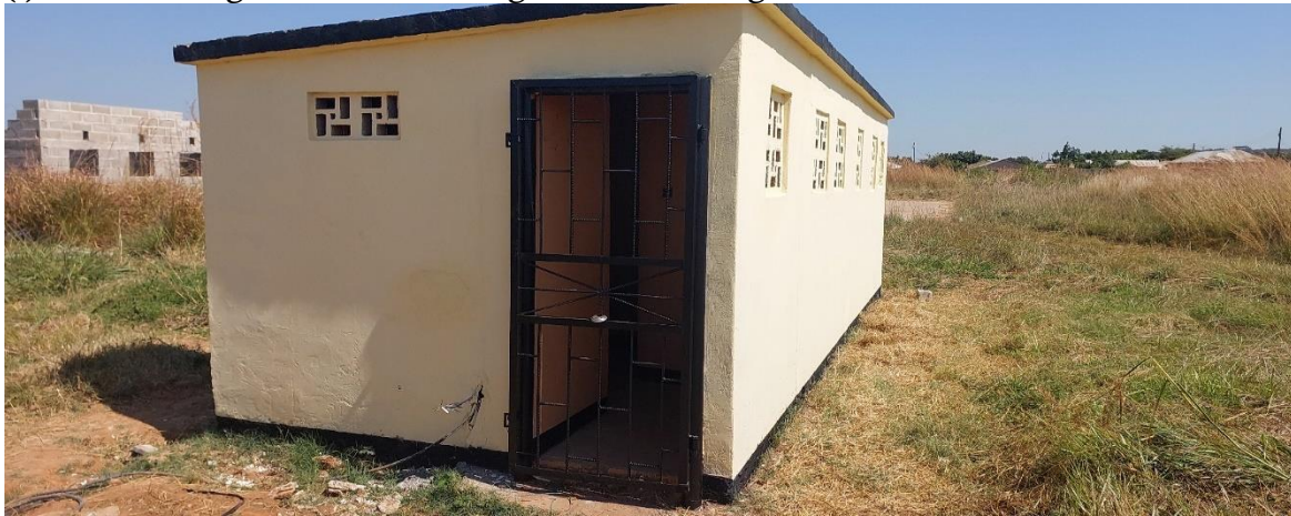
(ii) One of the two old ablution blocks being rehabilitated in place of the new ones whose funds were varied in order to construct the standard dressing rooms.
