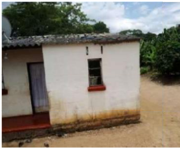
Dilapidated Low-Cost House
