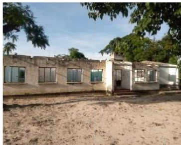
Dilapidated FTI – Sesheke
