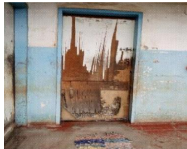
Worn Out Door
