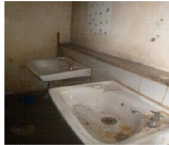
Dilapidated FTI – Sefula
