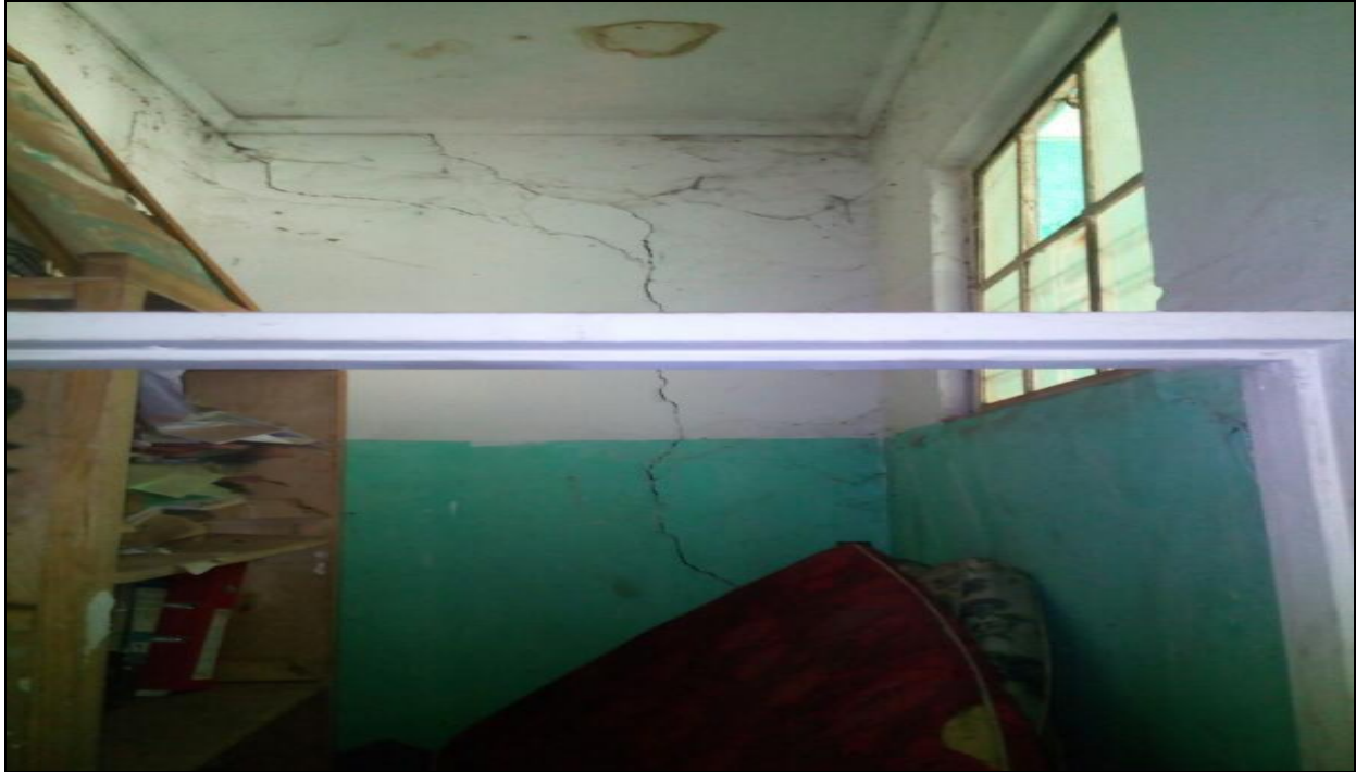
Cracked Livingstone DEC Office
