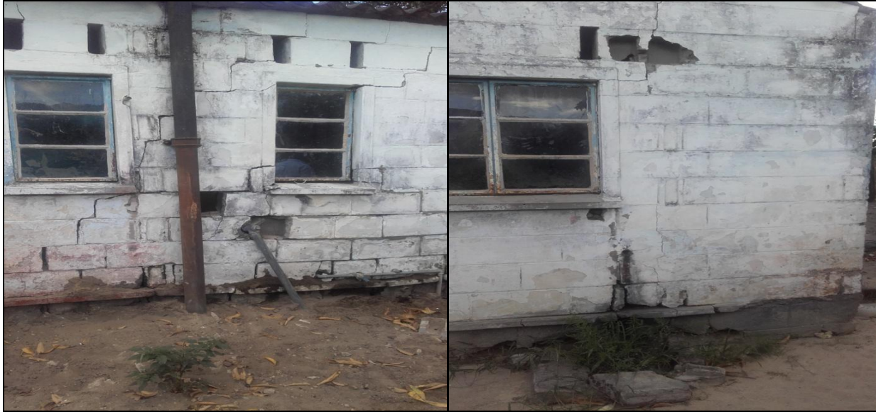
A dilapidated house in Mongu Police camp
