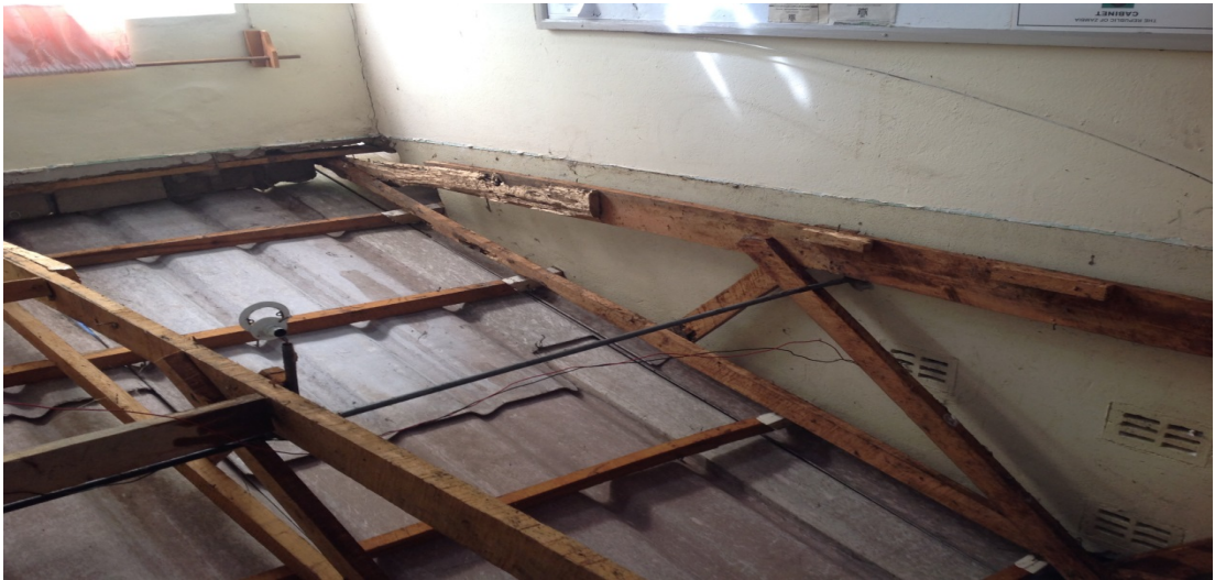
Picture 1: State of Provincial Administration building-Mansa
