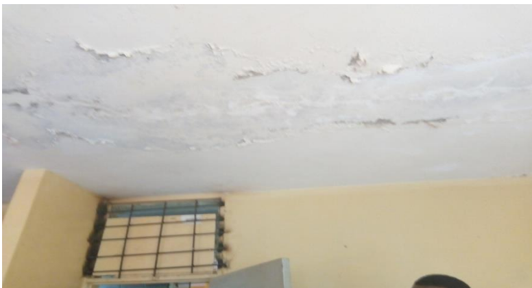
Fig.8: Leaking roof in the student hostel at NRDC
