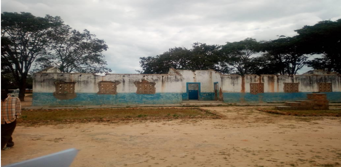
Current state of a 1X2 classroom block at Mateyo Kakumbi Primary school with blown off roof.
